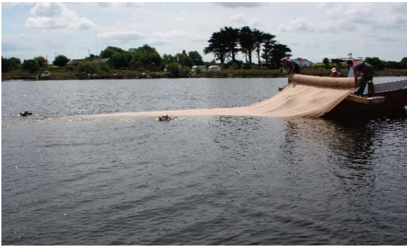
Laying jute mats in Lough Corrib to smother Lagarosiphon Photo: Joe Caffrey (IFI)
